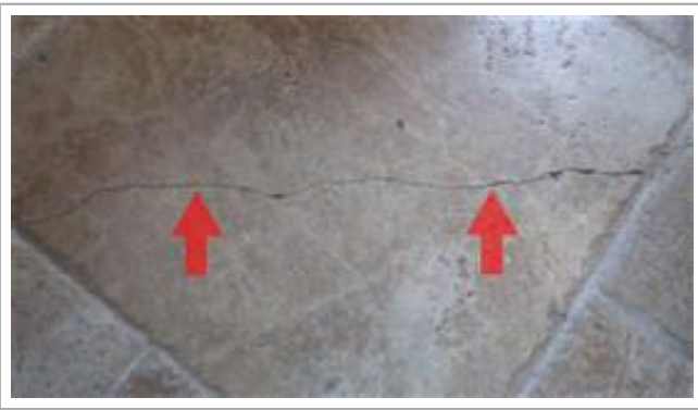
Common cracks noted in Master bath floor tile. No loose tile noted.
