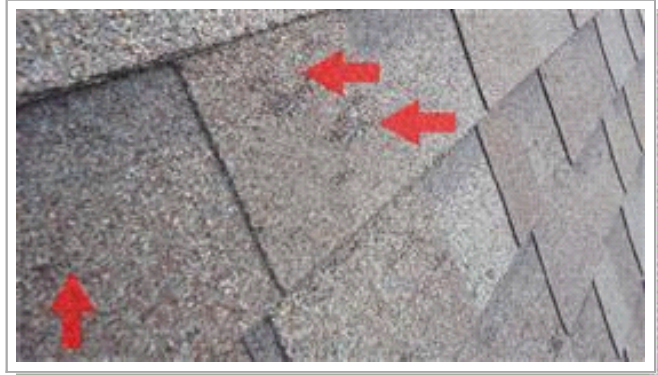
Extensive Hail damage noted on asphalt shingles at all four sides of hip roof.
