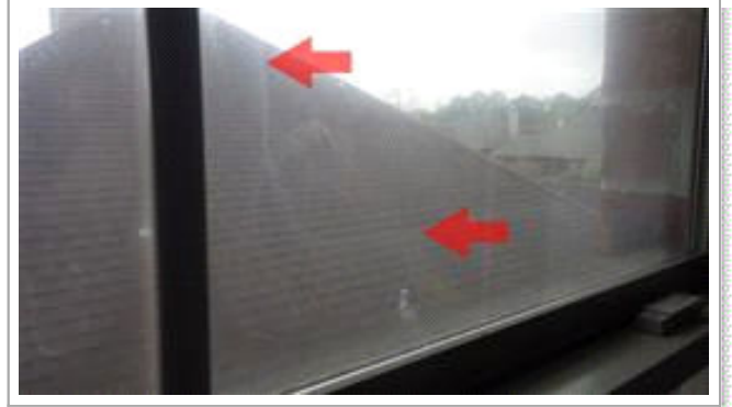
Failed window seal noted at 2nd level front bed room window. Condensation noted between the windowpanes.
