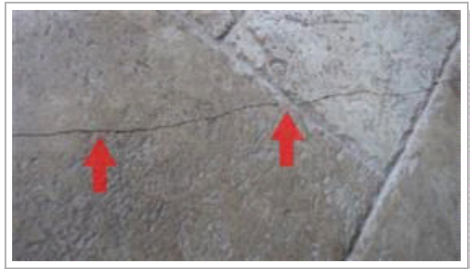
Common cracks noted in Master bath floor tile. No loose tile noted.
