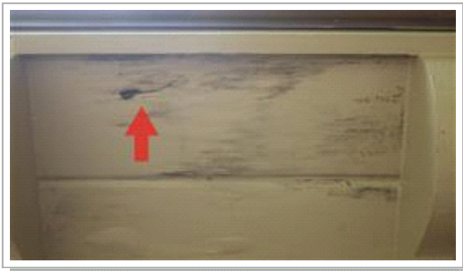
Minor wood rot noted on wood trim at right exterior eave.
