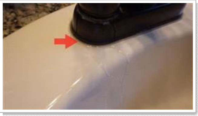
Water leak noted on faucet for 2nd level bath sink.
