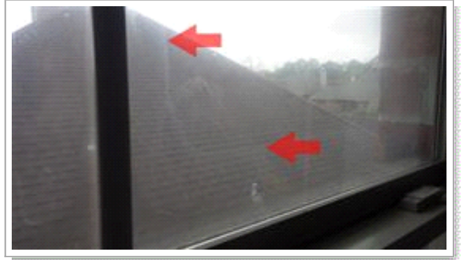
Failed window seal noted at 2nd level front bed room window. Condensation noted between the windowpanes.
