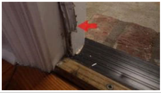
Damaged/Missing weather stripping noted at garage service door.
